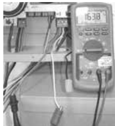
Figure 17. Output voltage measurement close up
