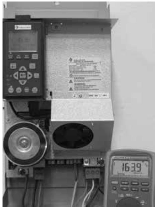
Figure 21. 3 phase 45Hz voltage measurement
